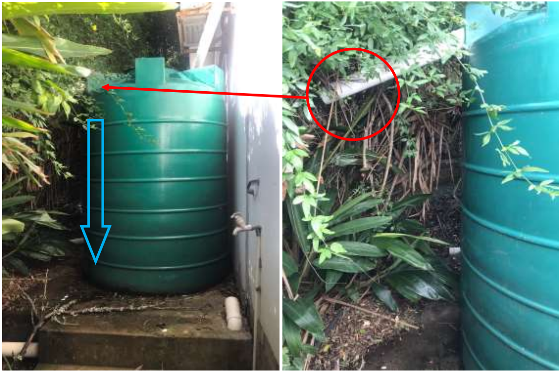
Tank discharge saturating soil
