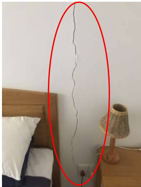
Crack in second bedroom corresponding to crack in next picture (corner bedroom)
